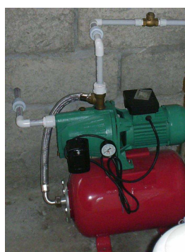
Pump and pressure tank
